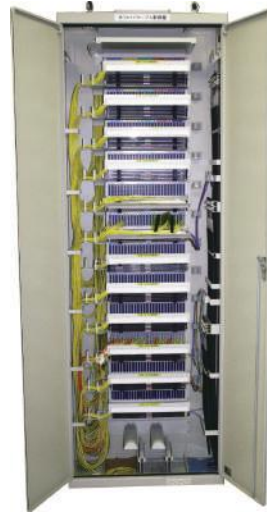
Standard type 2,400-port Termination Rack SC connector , Splice Tray
